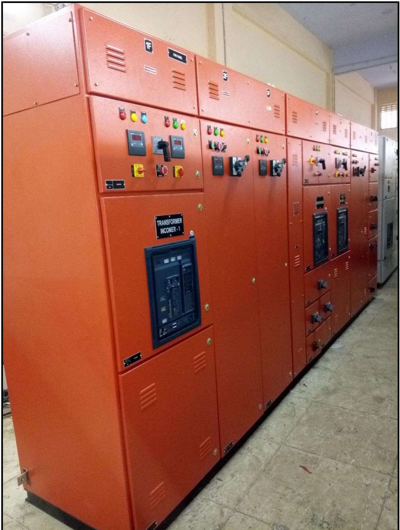
Fire Fighting Panel
